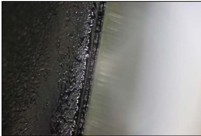
Figure 4- Tiny crack - detail.
